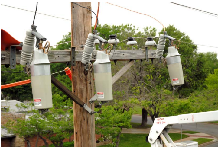
Oncor Electric Delivery
